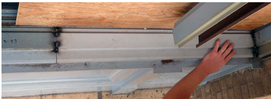
Photo of replacement section tack welded in place. There is a stainless steel backing plate that spans the joint. Welds will be made continuous along the joint and ground flat to the profile. Where required, epoxy patch material will be added.
